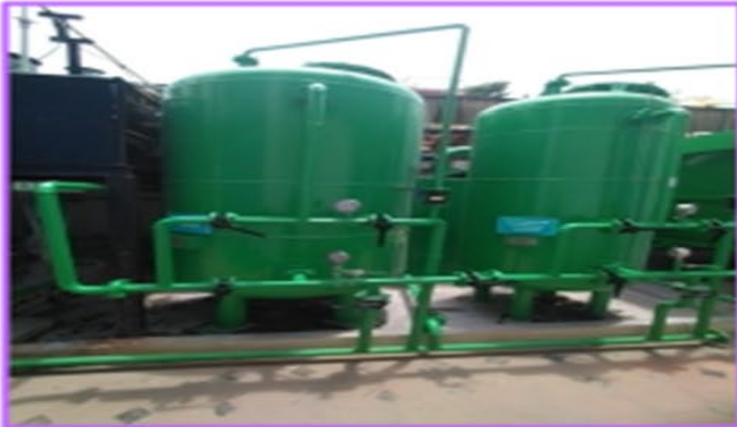
Glass and Activated carbon filter media
