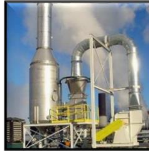
Wet scrubber – ventury type
