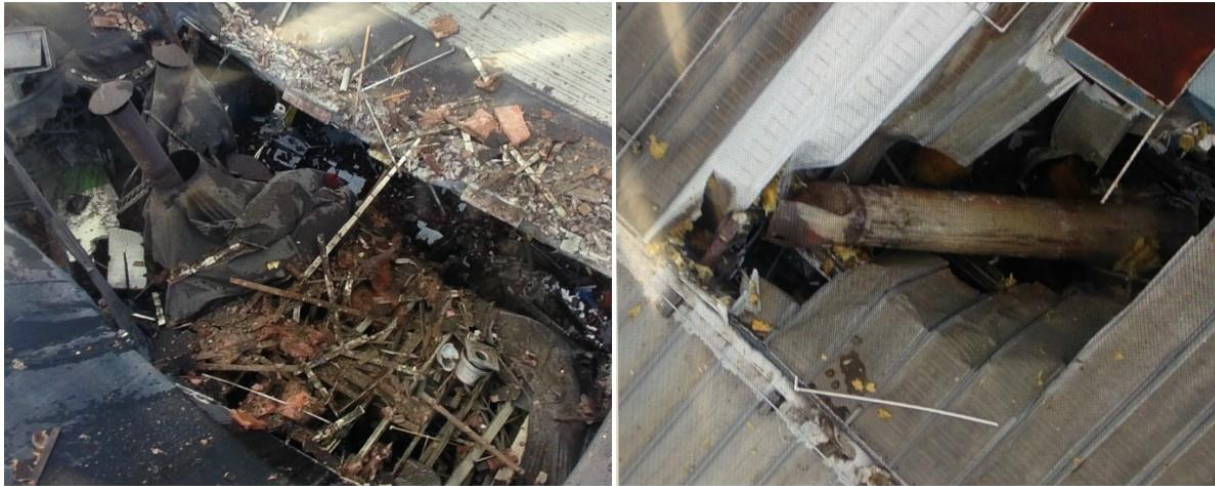
Images of facility after explosion
