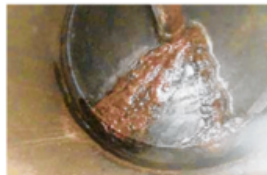
This photo, taken three days before explosion shows corroded tank bottom head.
