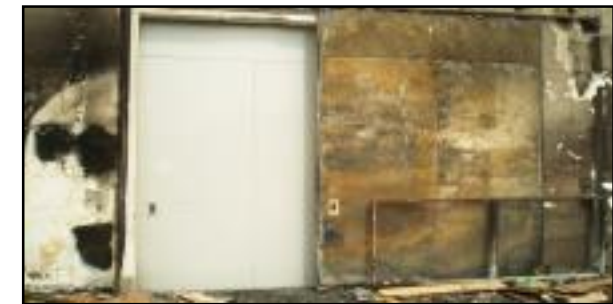
2 x 2 hours fire doors
