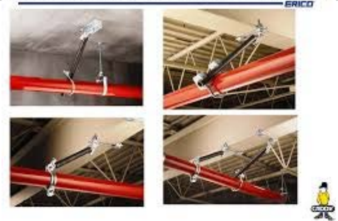
Fire Sprinkler Earthquake Protection – Sway Bracing
