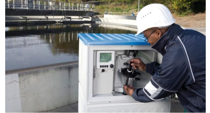
Typical composite sample installation
