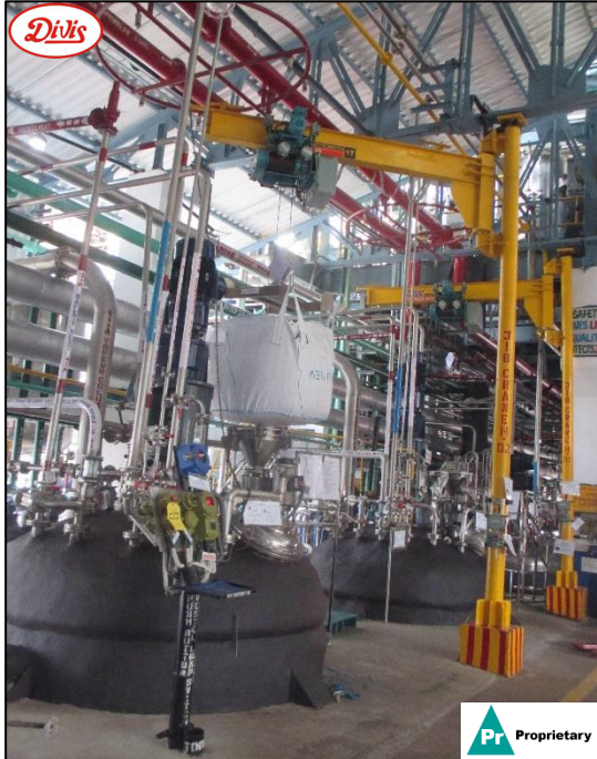
Big bag handling with JIB crane & Hopper
