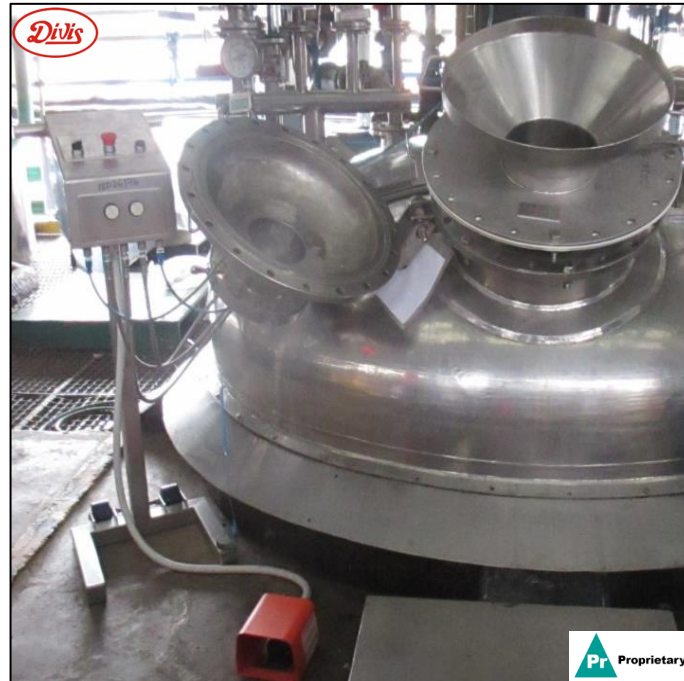
Charging through Manway purge hopper
