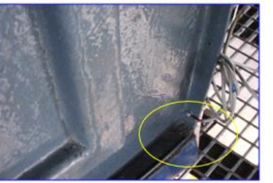
9. Ensuring the Grounding.
