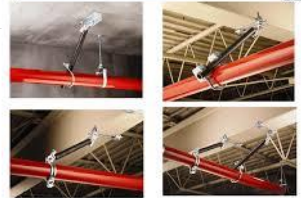
Fire Sprinkler Earthquake Protection – Sway Bracing
