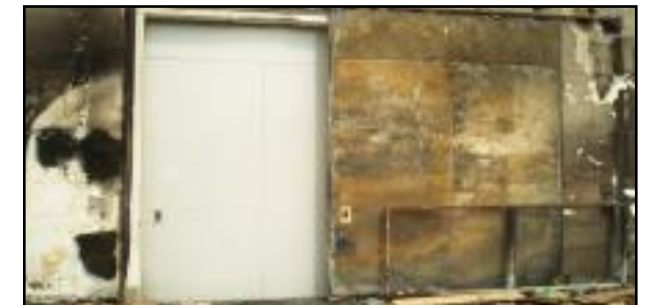
2 x 2 hours fire doors
